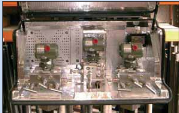
IEX3 Enclosure with heating system and insulation
